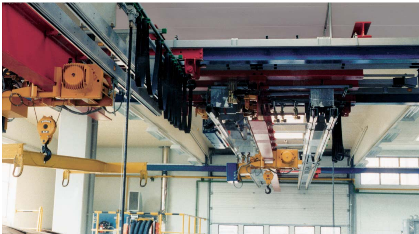
Aluminium enclosed conductor system on crane bridge.
