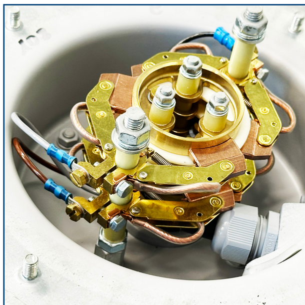
the view inside the sliprings compartment side
